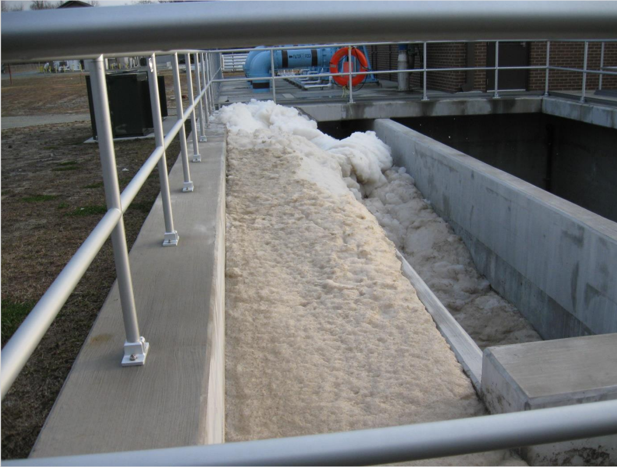
Filter influent channel
