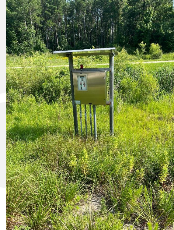
LEACHATE PUMP STATION
